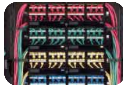
Covers are included with the cable managers to provide a clean patching appearance.
